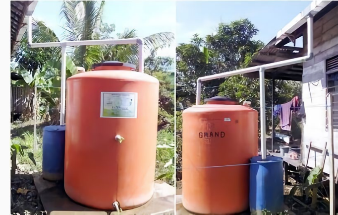
Rain water harvesting
