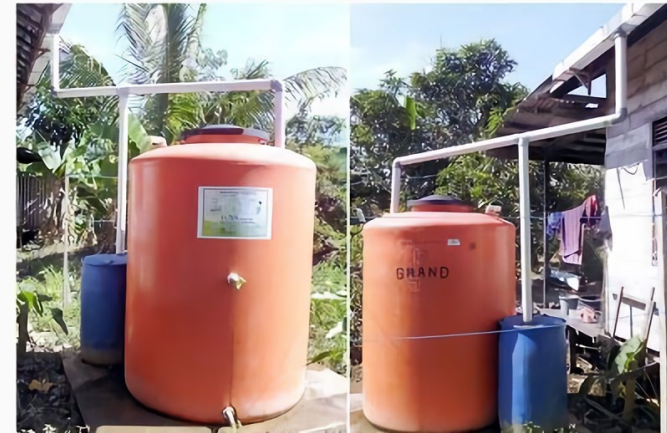
Rain water harvesting
